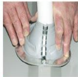
5 Snap on the required number of additional clips and crimp closed. Apply Sealant between Zip Seal base and roof sheet
