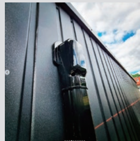
Photo provided by JMG Cooling Services (UK)
